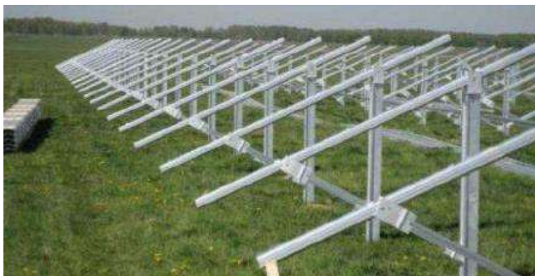
Structures de support sans modules
