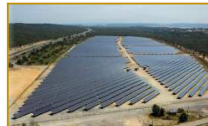
Rochefort-du-Gard – 11 MWc Friche naturelle
