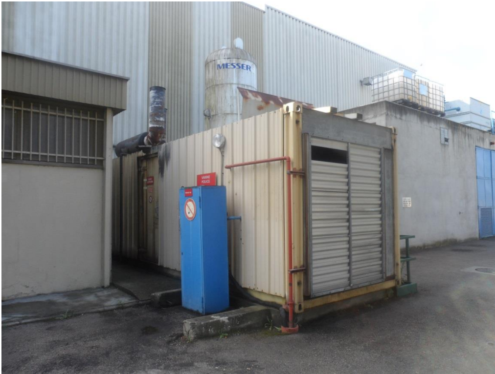
Photo zone 4 & 5– local sprinkler
